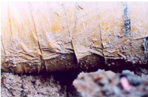
Soil Stress Failure
